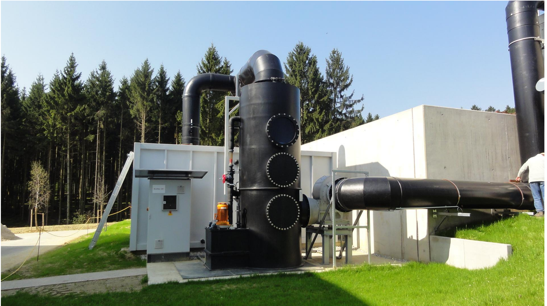
Exhaust air scrubber with biofilter
